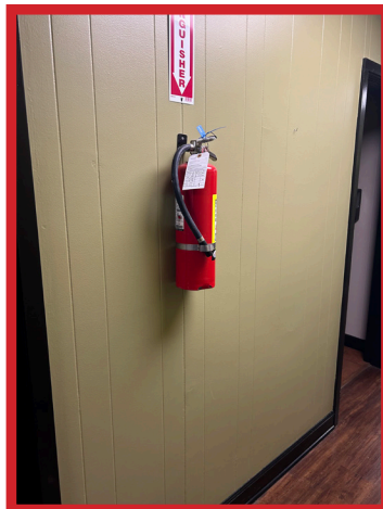
Fire extinguisher needs to be lowered and braille signage
