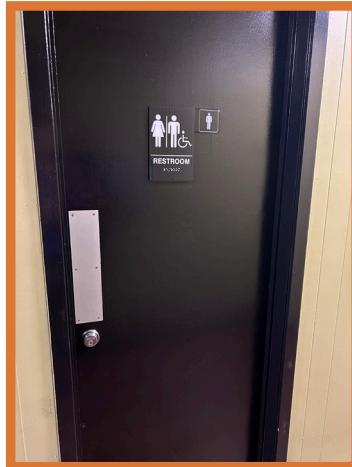
Sign placement is non-compliant
